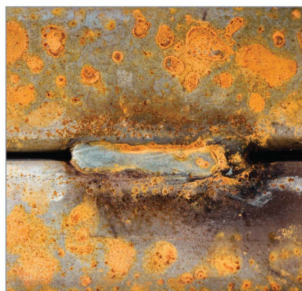
OVERLAPPING SURFACES. Leave minimum gap of 2mm between overlapping surfaces. Where seal welding is not practicable stitch welding should be used.
